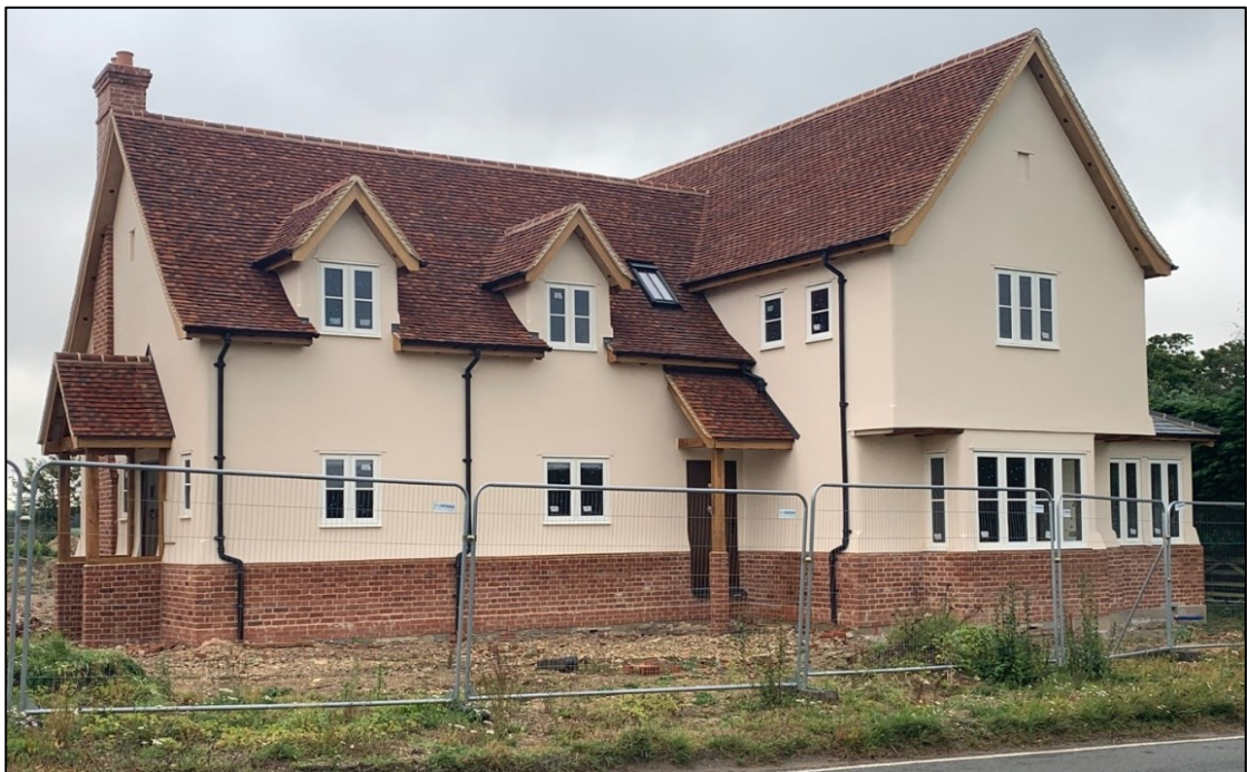
Figure 16: Homes under construction at Well Court in Hunsdonbury reflect roof lines and dormer features
